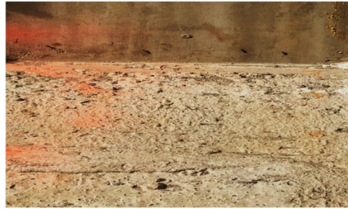
Figure 6: unacceptable substrate concrete protrusions
