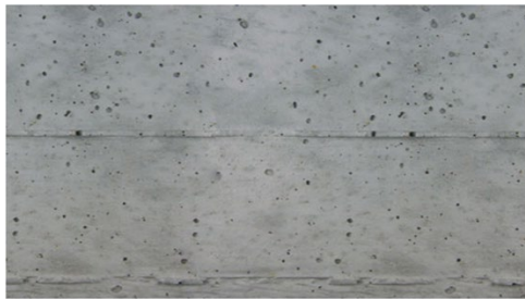
Figure 7: unacceptable bug holes and fins
