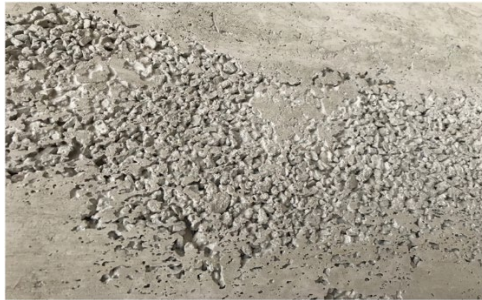
Figure 5: unacceptable substrate honeycombing
